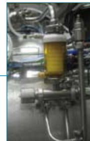
DECONTAMINATION OF EXHAUST AIR WITH STERILE FILTER
