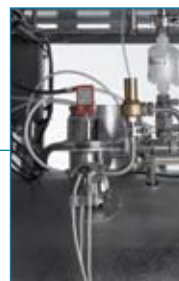
MODULATING VALVE ON FEED STEAM INLET
